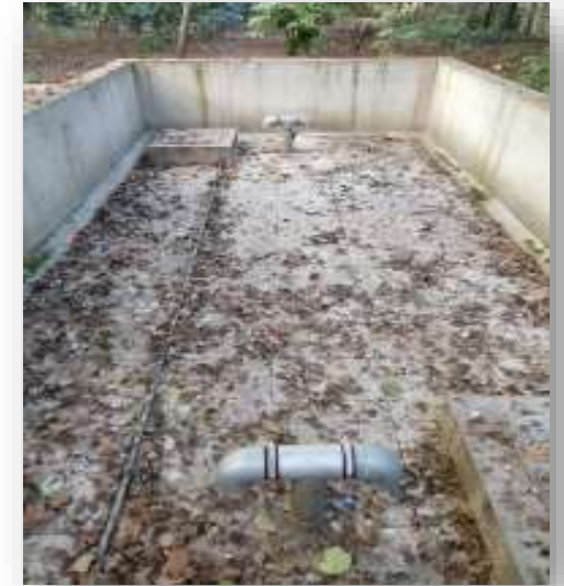
Rainwater Harvesting Sump
