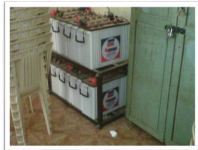
Power back-up in the Computer Lab
